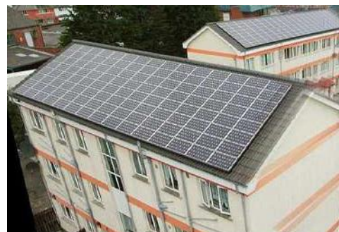
Figure 3. Solar PV added to roof.
