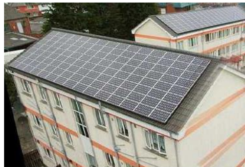
Figure 3. Solar PV added to roof.
